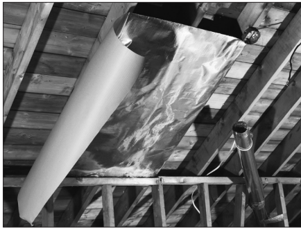
The Oak Ridge National Laboratory estimates that installing radiant barriers can save about $150 a year in hot climates and $40 in cold climates.
